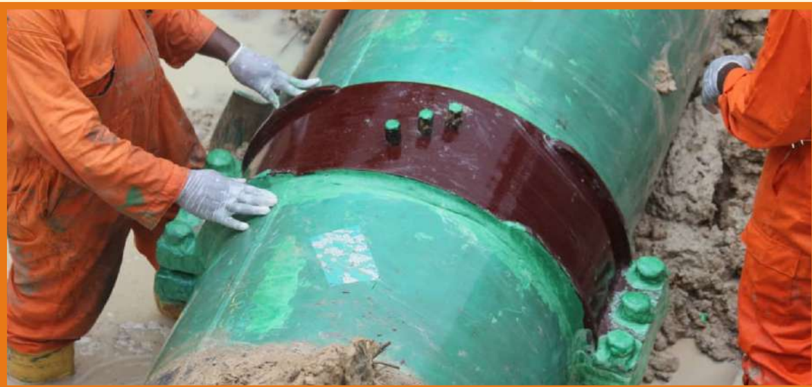
30" West Africa Gas Pipeline Leak Repair
