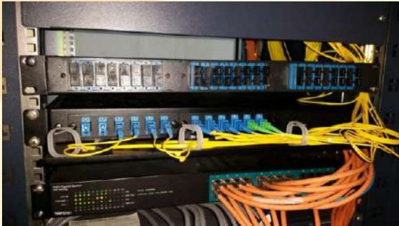
Access control & monitoring systems configuration & training
