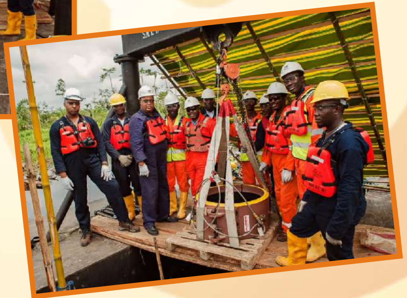
30" West Africa Gas Pipeline Leak Repair
